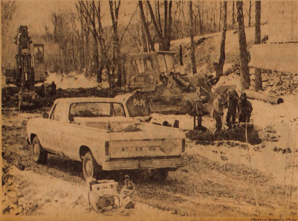
Workmen from the Ben Construction Co., one of the contractors on the Franklin Township Sewer project, put the finishing touches on the last of the collector and interceptor lines.
