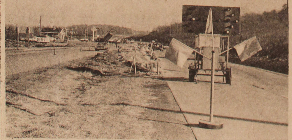
Two contractors work on Route 21 crossovers just east of the Greene Plaza Shopping Center near Waynesburg. Observer-Reporter Photo
