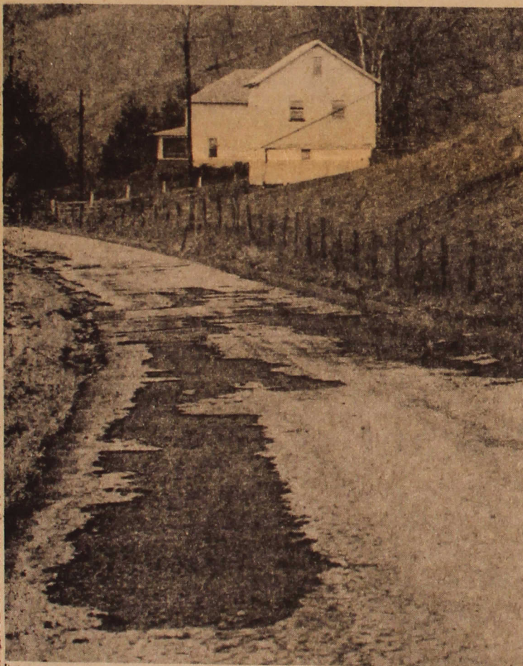
Portions of road between Oak Forest and Kuhntown were washed away.
