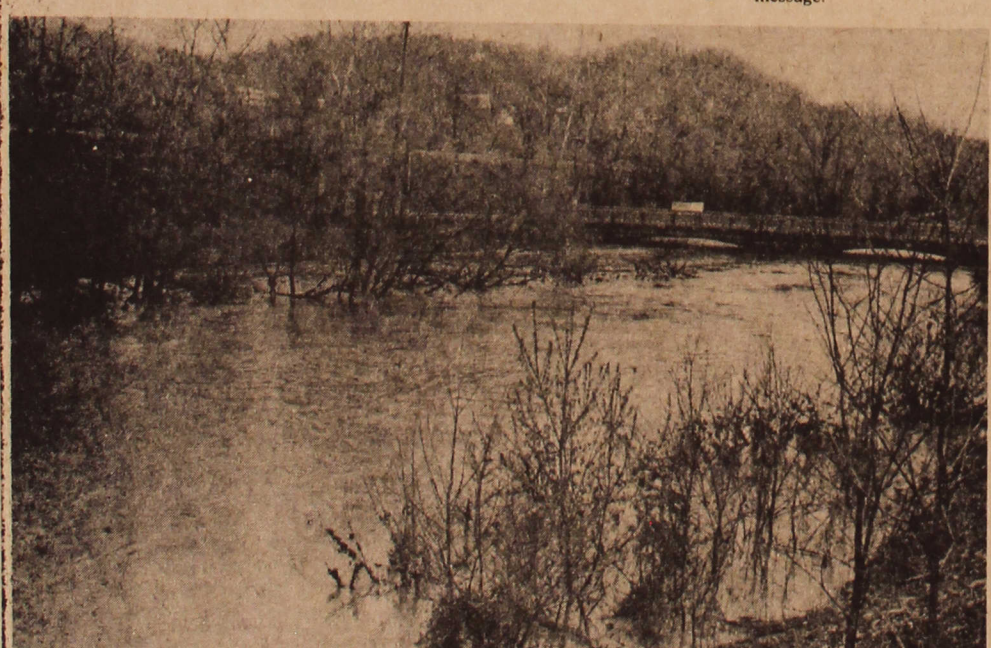
Monday morning water was still close to the bridge deck that carries Routes 19-21 over Ten Mile Creek just east of Waynesburg.
