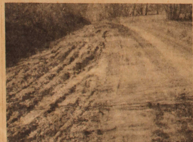
Ruts in Route 30081 in Morgan Township.
