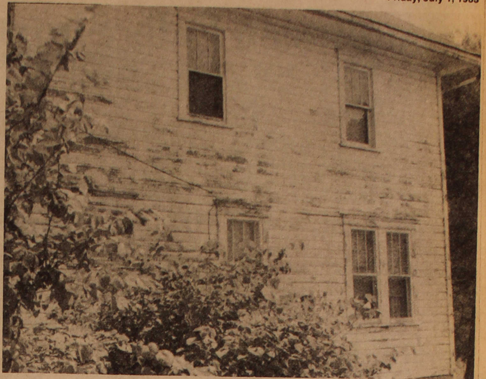
One of the houses in Blairtown with peeling paint
