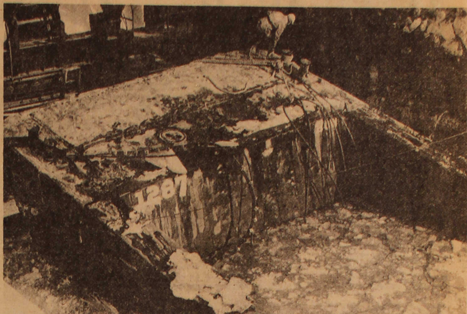
Workman attaches cable to floating section of barge in Monongahela River near Pt. Marion.
